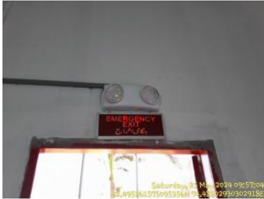
Emergency Exit Sign with Light.jpg
